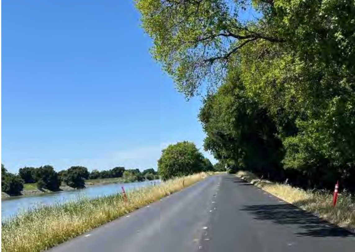
Road maintenance is happening now on River Rd along the Sacramento River, between the town of Locke and Twin Cities Rd.
